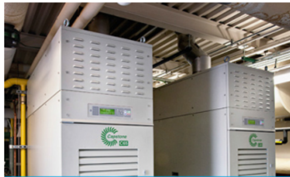
Microturbine CHP installation at a commercial facility. Photo courtesy of Capstone Turbine Corporation
